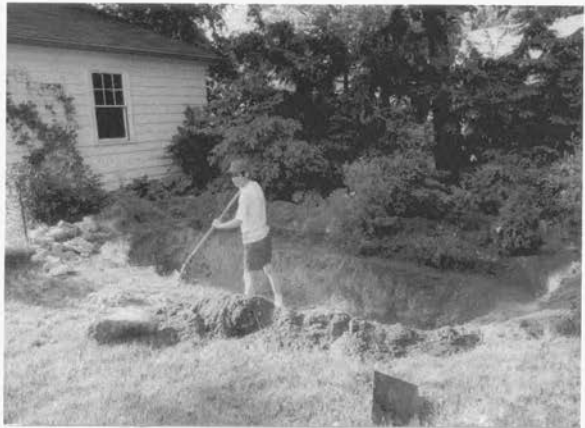
Figure 1. Excavation of the pond in progress, showing the basin and the shelf around the edge (photographs by the author)
